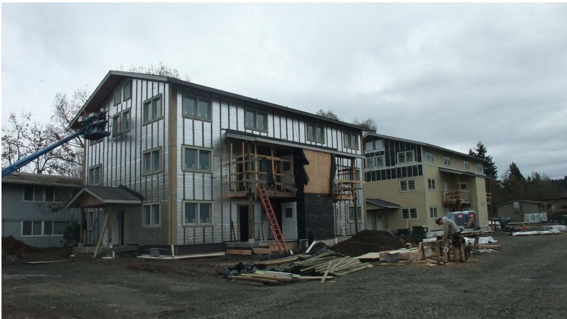
Figure 2: Continuous insulation over WRB on PH (left), siding directly over WRB on EA (right) (Author 2013)
