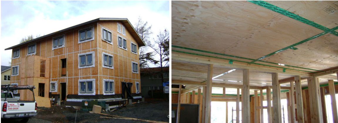
Figure 4: Taped plywood seams throughout PH (Author 2013)
