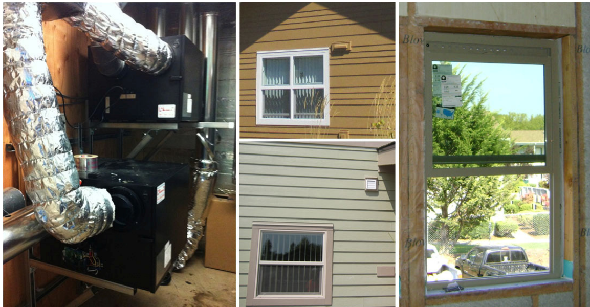
Figure 6: ERV at PH (left), examples of passive air inlets (center), trickle vent at window head at EA (left: Kwok 2014, center and right: Author 2013)
